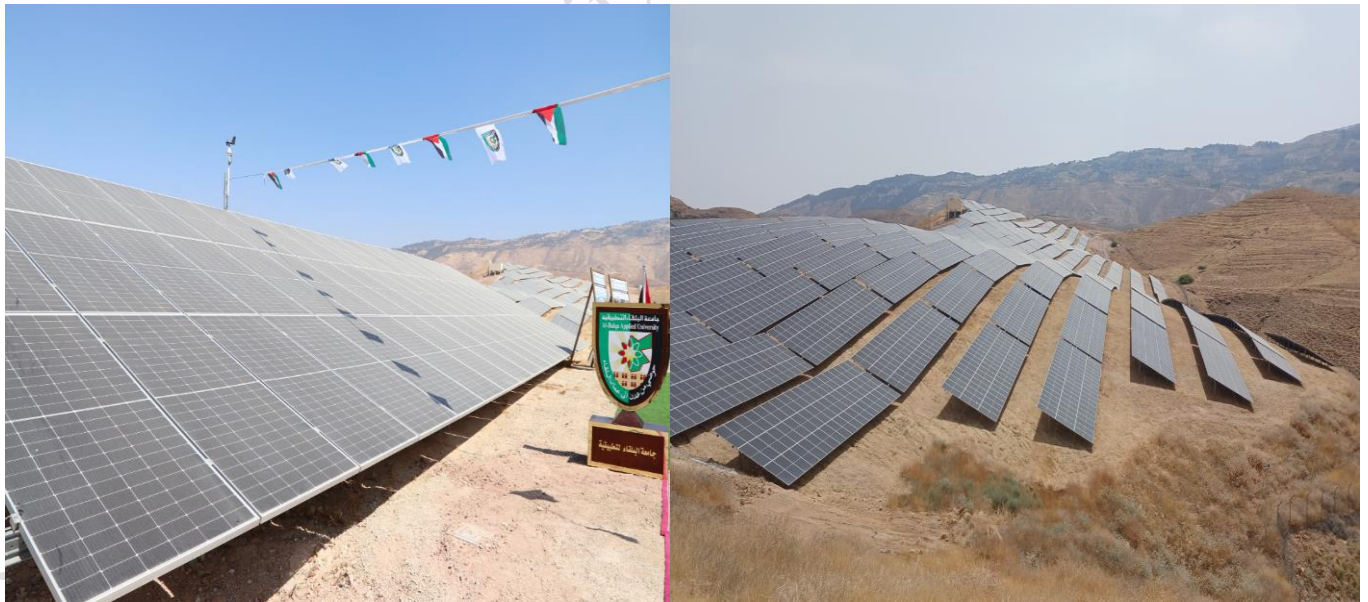
BAU's Solar park project with capacity 7MW
